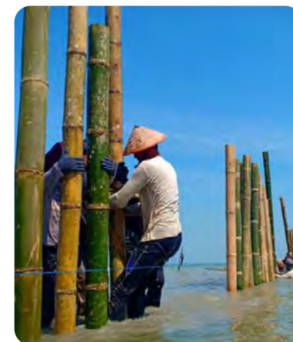
Community members work together to construct a permeable sediment trapping structure in Timbulsloko Village, Indonesia. © Kuswantoro
